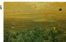
Example of Powderpost Beetle Damage
