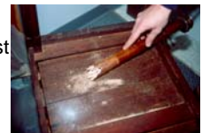
Example of Lyctid Beetle Damage
